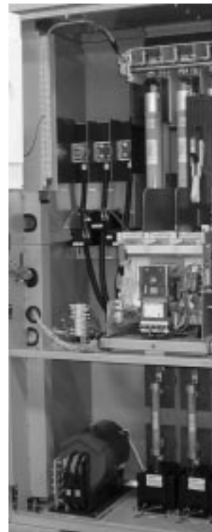
15 kV AMPGARD Starter — Medium Voltage Door Open
