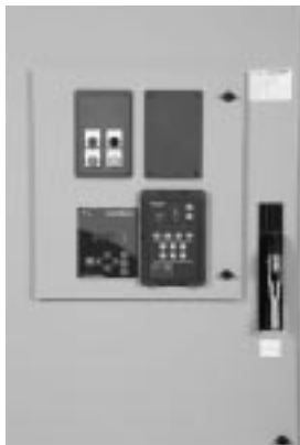
Low Voltage Door with InsulGard Relay
