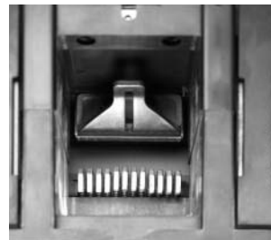
Magnum DS Breaker Contacts (Arc Chutes Removed)
