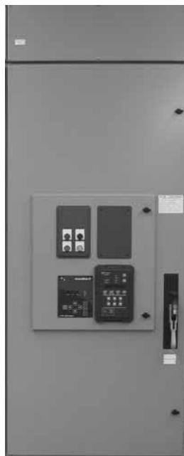
15 kV Starter with InsulGard
